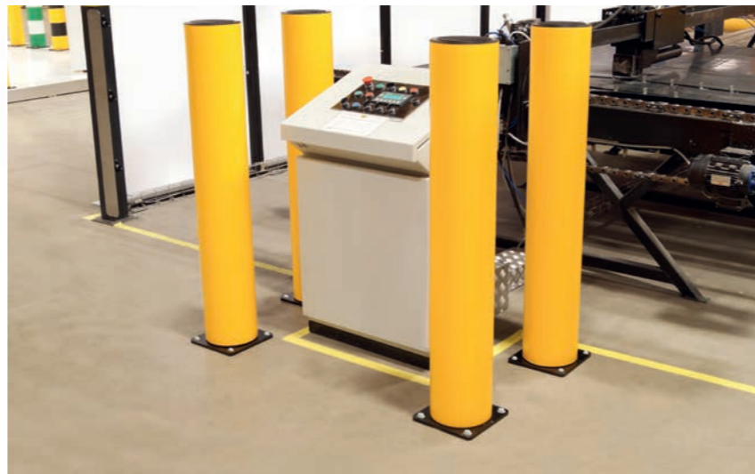
Allow constant access to frequent-use machinery and equipment, whilst protecting from impact with a high strength visual alert.
